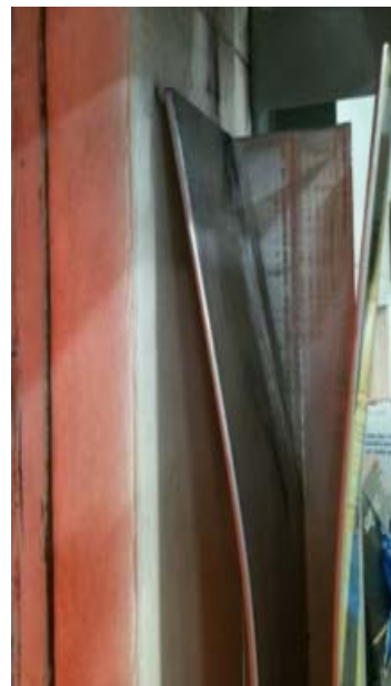
Top Track Adjustment for curtain entrance
